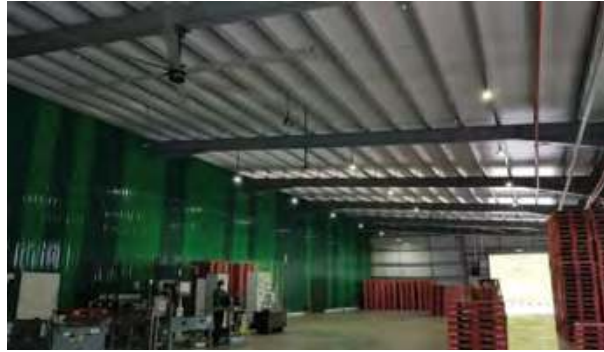
HVLS fan installed at pallet inspection area
