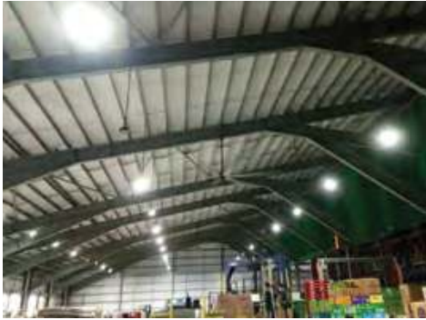
LED lowbay light at staging, pallet inspection & racking system
